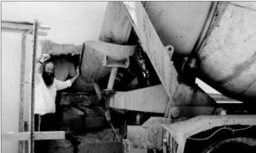
On the scene as cement is poured at the mikva in Kfar Chabad Beit
